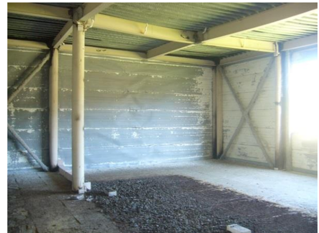
Fire load after the test
